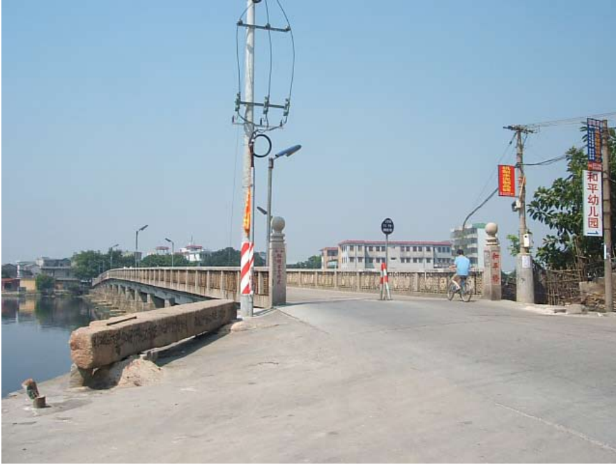
FIGURE 1. Heping Bridge in Chaoyang. Photographs on this page and the next were taken by the author in July 2008.
